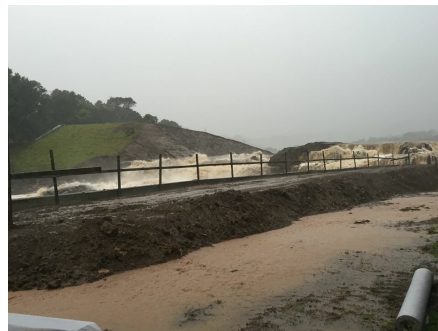
<— Water rushing through hole cut in dam wall behind concrete wall built to protect the Centre
